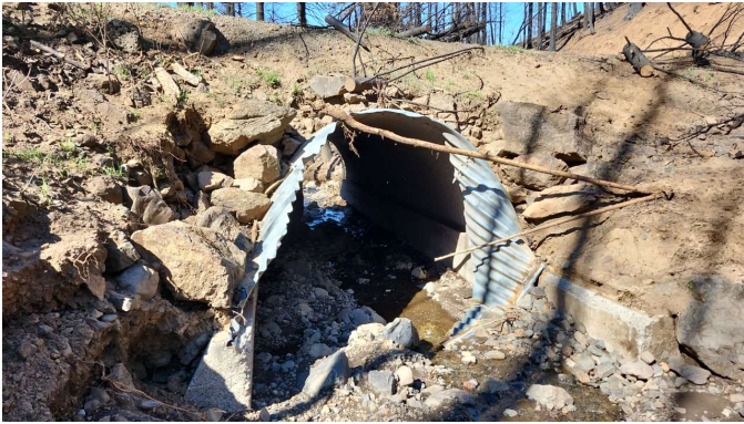
Figure 4. Culvert damage from post-fire flooding
